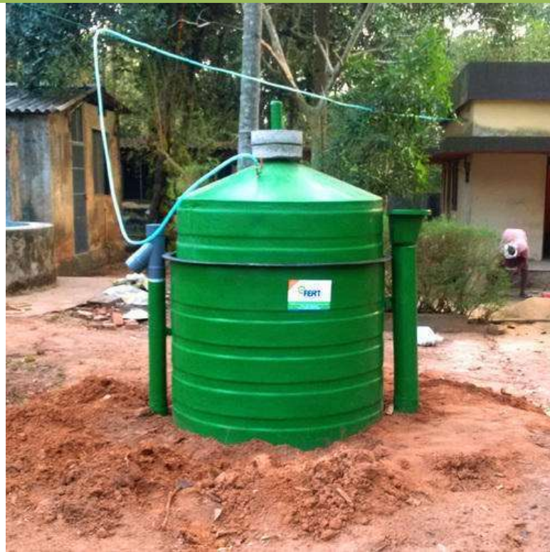
Bio-Gas Generation Plant - 10g/day- At canteen
