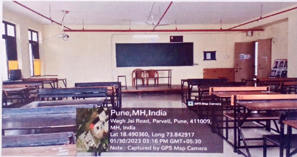
Classroom showing LCD Projector with LAN (Room No. 127)
